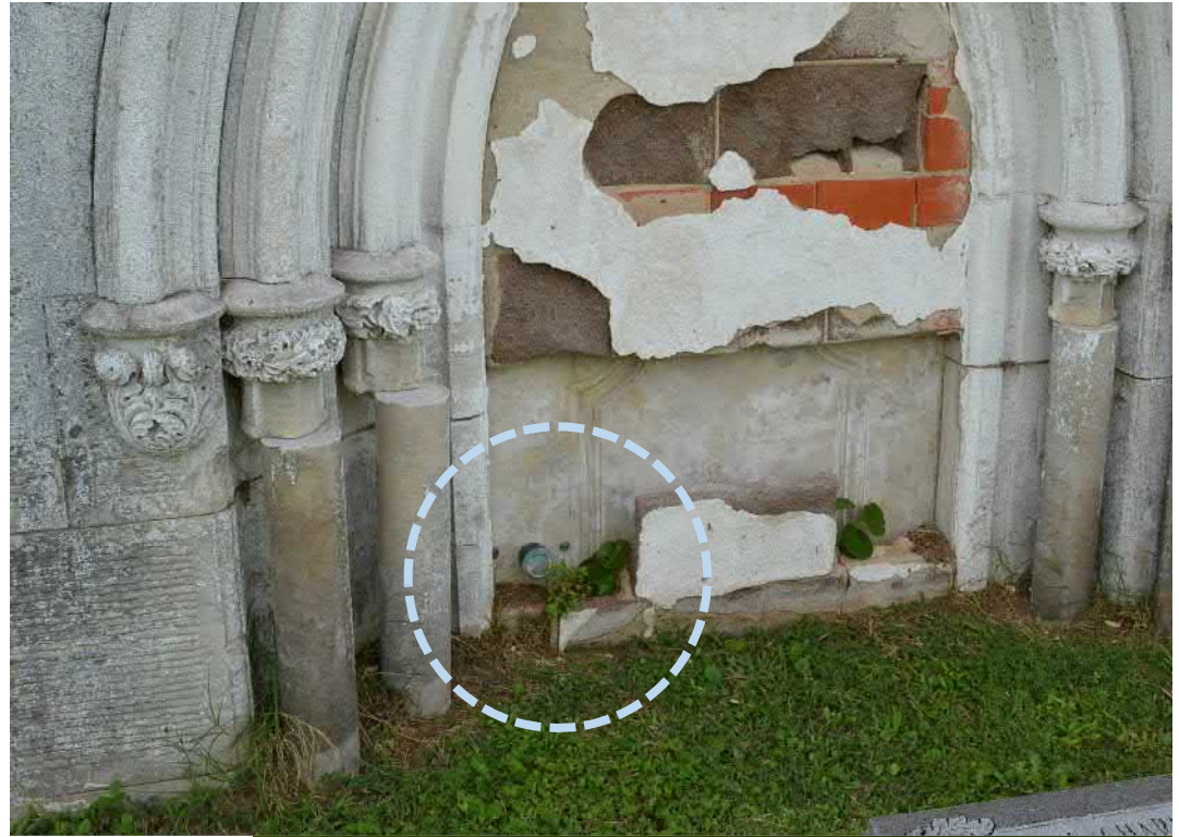
Broadway Cemetery, Episcopal Section, Galveston Ground level raised in late 19 th century resulting in a partially covered doorway.
